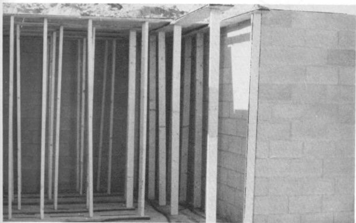
Fig. 9-4. Wood against the floor is not glued in place.
